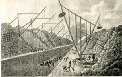
Section of Erie Canal, one thousand feet, West of Lockport This "mountain ridge" was considered the most difficult work of the original canal. Here was struck the last link just prior to the celebration at the formal opening on October 26, 1825. From a print in Colden's Memoir.
